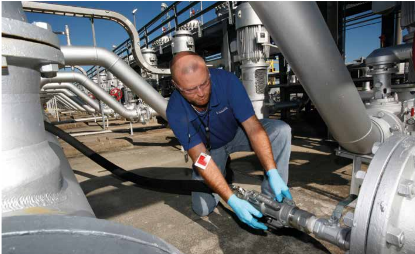
Today's advanced dry disconnects have been designed to reduce connection time from 30-40 minutes to just 30-40 seconds
