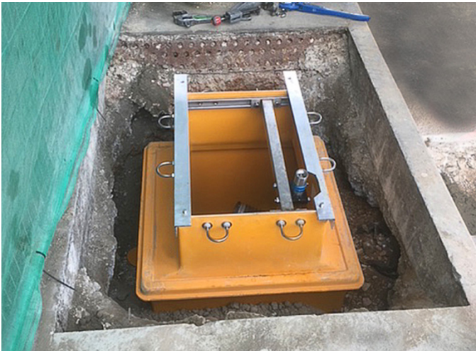
BP required retrofit chamber systems
