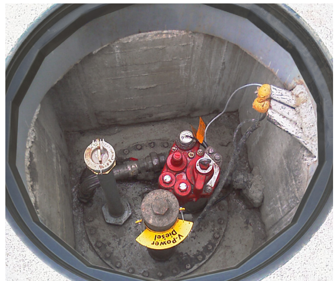
Fibrelite's covers prevented surface water ingress into chambers above the fuel tanks
