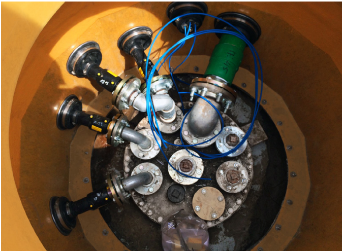
OPW provided a long-lasting containment system
