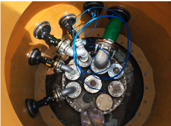
OPW provided a long-lasting containment system
