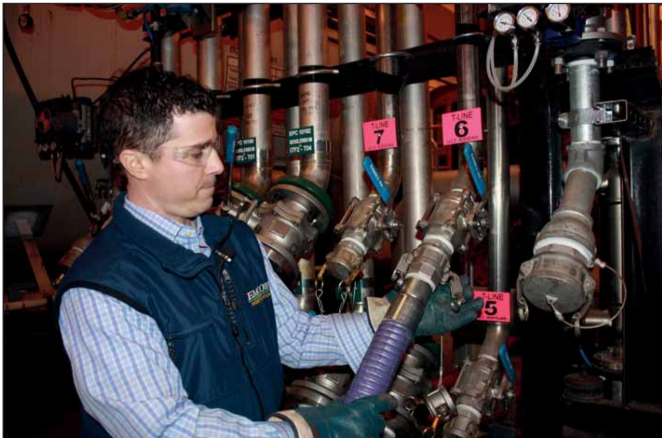
With the different types and large volumes of chemicals that the new EMCO facility handles, VP Engineering BJ Korman needs dry and quick disconnect couplings that are both highly reliable and easy to operate
