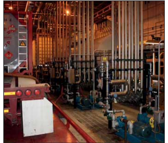
EMCO's side-by-side tank-truck and railcar loading/unloading dock features numerous loading racks that are dedicated to specific products or raw materials.
