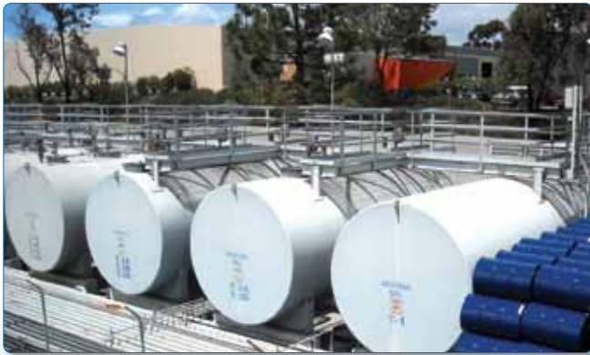
OPW's SiteSentinel® iSite™ ATG system was installed on 32 ASTs at SKS Oil's bulk-lube storage facility.
