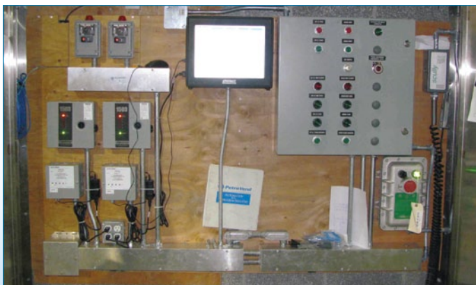
The control panel designed by P.D. McLaren features the OPW SiteSentinel iSite automatic tank gauging system.
